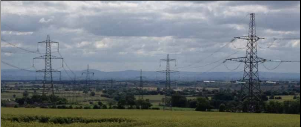
Figure 5.4 Suspension Tower (left) and Tension Tower (right)
